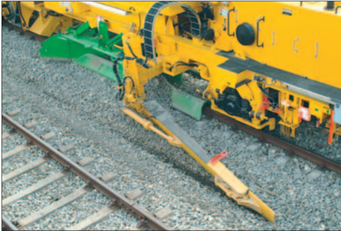
Fig. 9: Profiling and shoulder plough on the SSP 110 SW ballast-distribution and profiling machines
