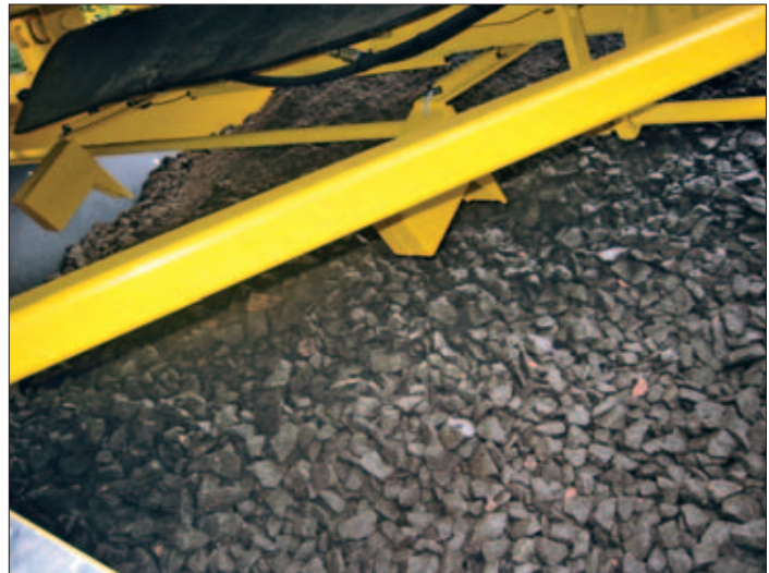
Fig. 6: Belt control for MFS material conveyor and hopper unit
