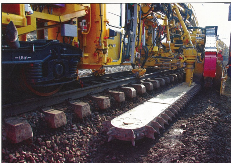
Fig. 3: The ballast excavation chain can easily be inserted underneath the track panel following removal of the shoulder ballast – no track panel dismantling or access hole digging is required
