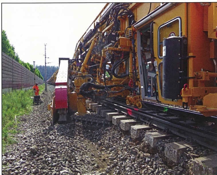
Fig. 4: Soiled ballast that has been removed from underneath the track panel onto the shoulder area is continuously picked up by the scraper conveyor system and transferred to the ballast screening unit for cleaning
