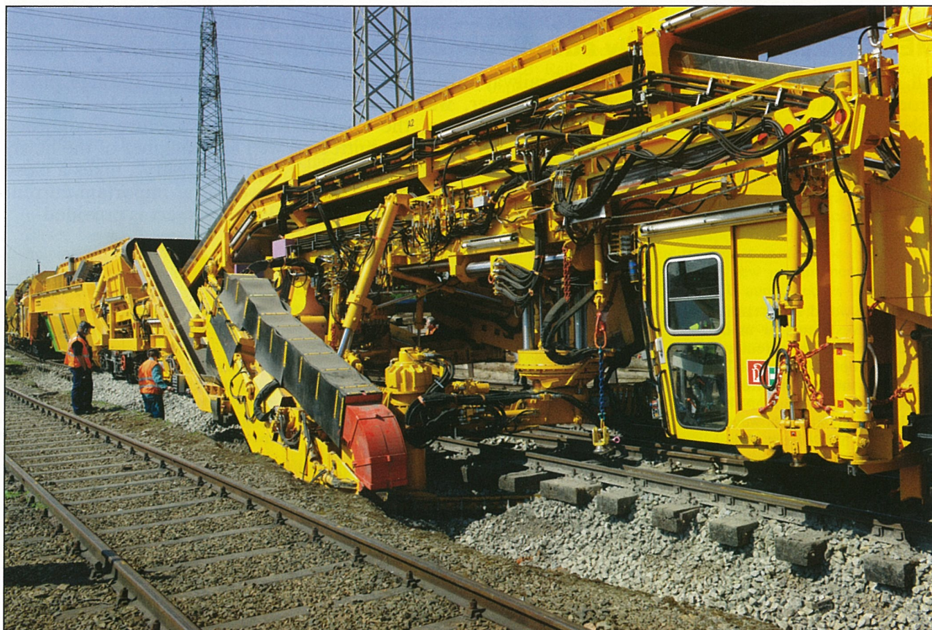
Fig. 5: Efficiency of the URM 700-2 in action: whilst the soiled ballast material is being removed, the cleaned or new ballast is already deposited directly behind the ballast excavation unit – a high-quality delivery geometry of the turnout is thus achieved
