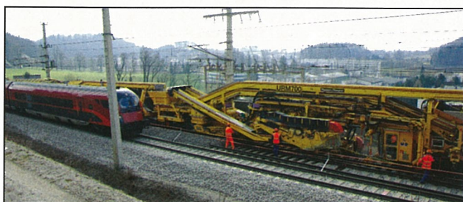
Fig. 2: No traffic disruption on the adjacent track – machine operations solely take place on the track under repair, without infringing the clearance gauge of the adjacent track
