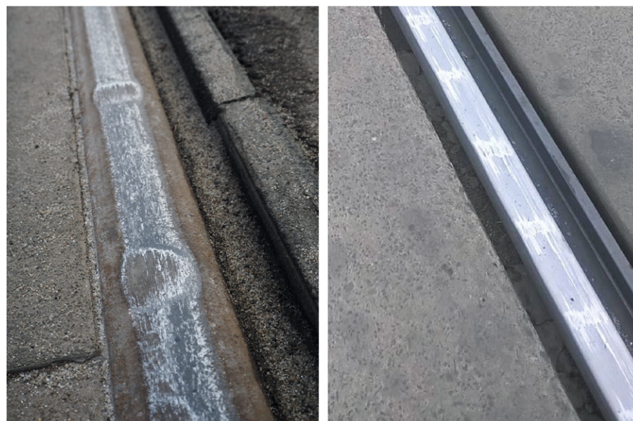
5: Common rail defects for grooved rails: Wheel burn (left) and corrugation (right)
