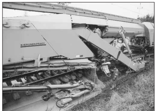
Fig. 3: Excavation of material and simultaneous installation of a compacted formation protective layer
