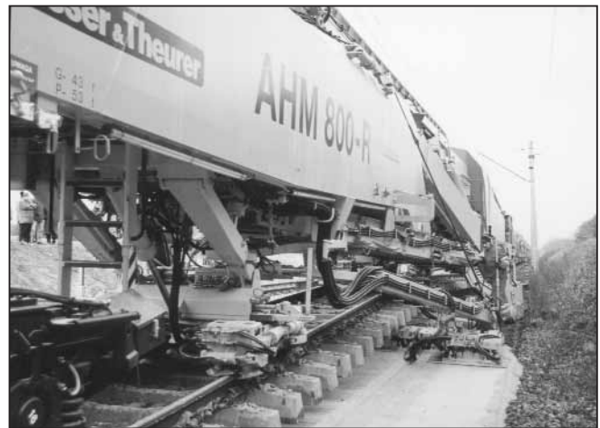
Fig. 2: Raising the track and insertion of the new formation protective layer without dismantling of the track skeleton, using the AHM 800-R
